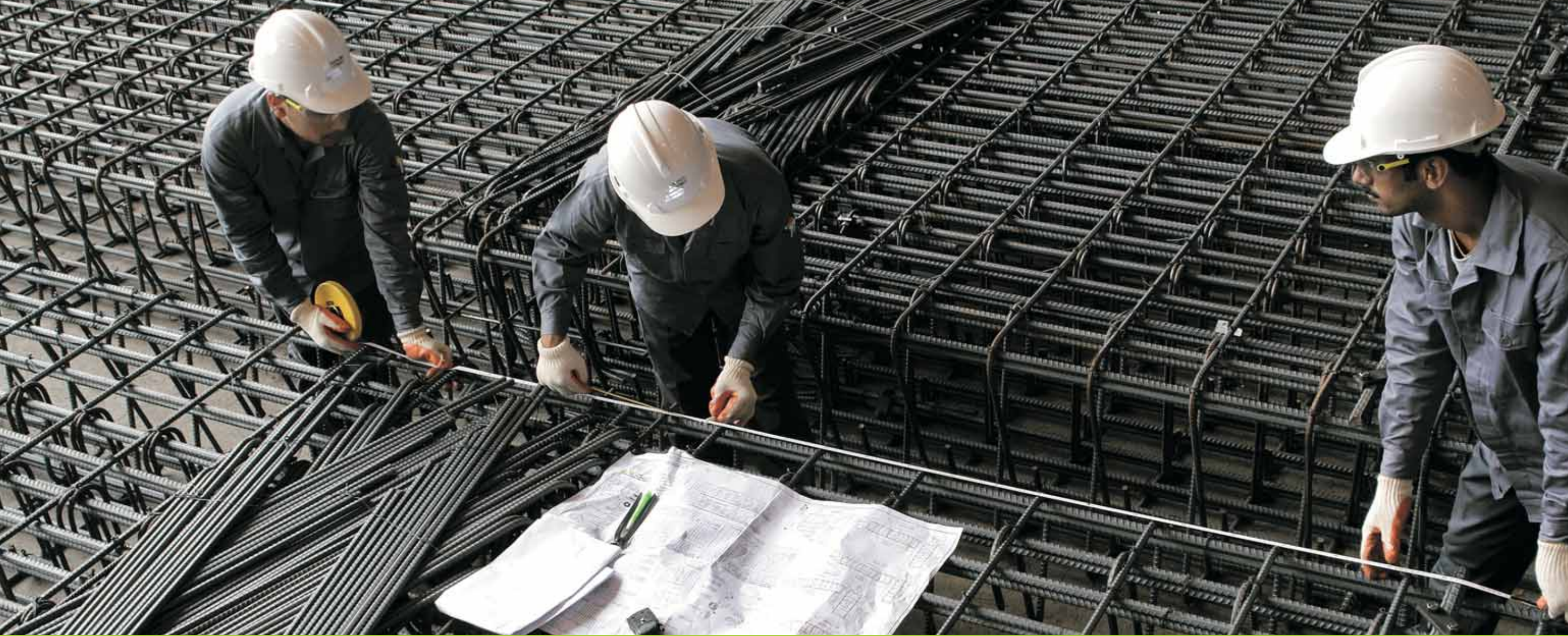
Prefabricated diaphragm wall cages of consistent quality and accuracy provide ease of installation and faster construction.
